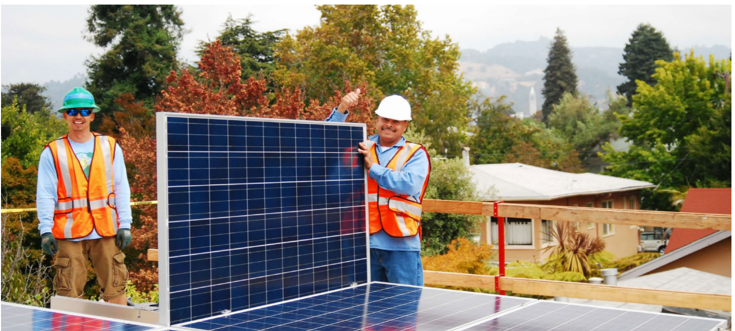
Technicians install solar panels at Unity Gardens, an affordable housing property owned and operated by Northern California Land Trust in Berkeley, CA. Photo credit: RE-vol.
