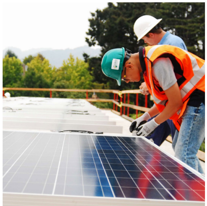
Technicians install solar panels at Unity Gardens, an affordable housing property owned and operated by Northern California Land Trust in Berkeley, CA. Photo credit: RE-volv.
