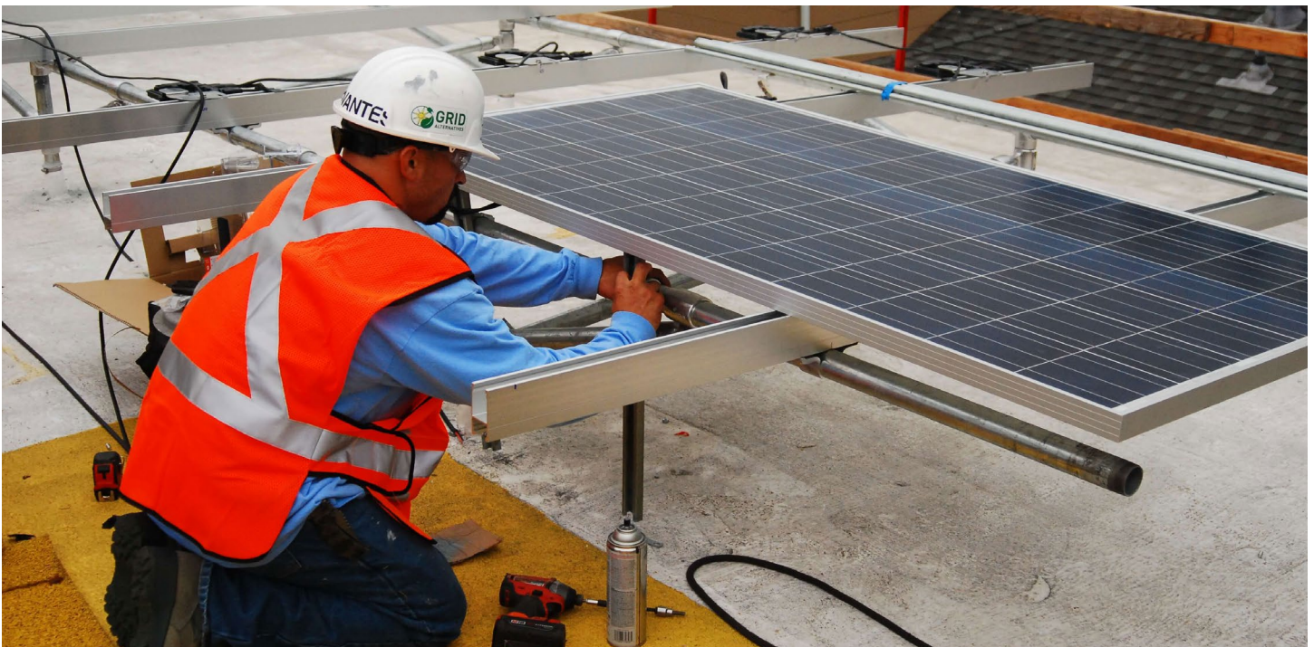
Technicians install solar panels at Unity Gardens, an affordable housing property owned and operated by Northern California Land Trust in Berkeley, CA. Photo credit: RE-volv.
