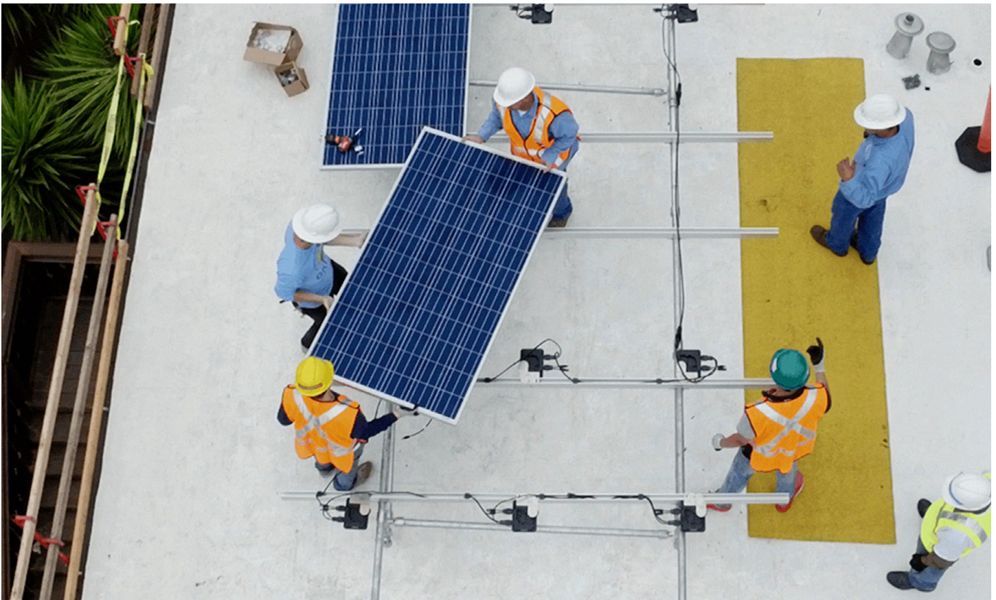
Technicians install solar panels at Unity Gardens, an affordable housing property owned and operated by Northern California Land Trust in Berkeley, CA. Photo credit: RE-volv.
