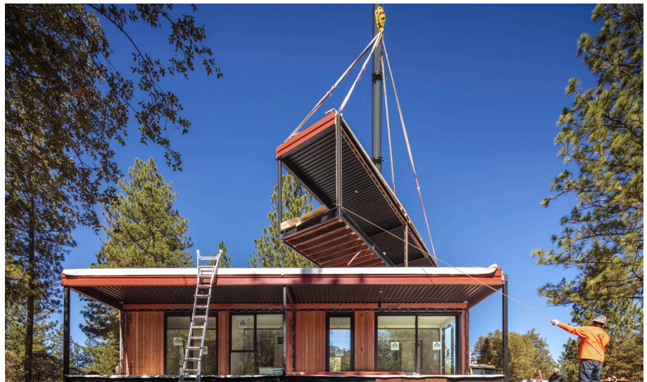
New housing module lifted into place by crane on a Connect Homes market-rate house
