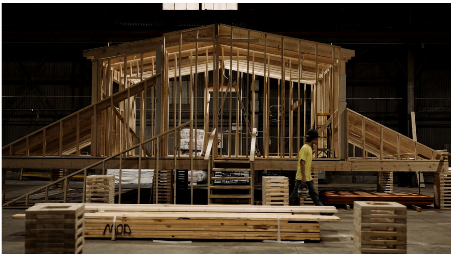
A Module home under construction at the Last Mile Facility in Carnegie, Pennsylvania
